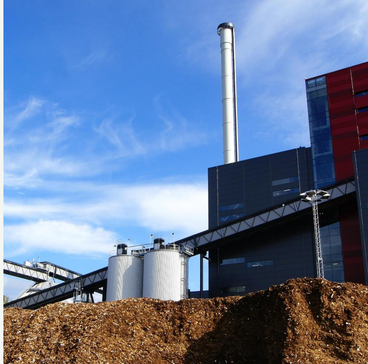
Fig. Biomass power plant
